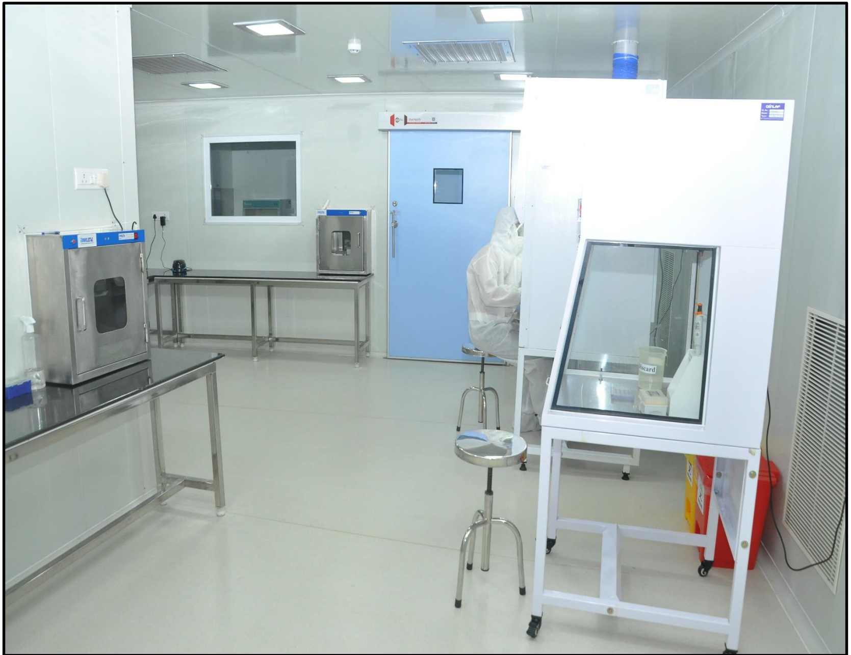
Extraction Room with Negative Pressure
